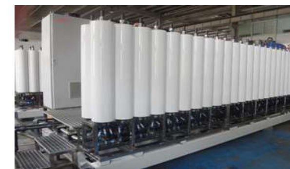
DTRO for leachate wastewater
