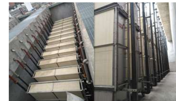
FMBR for industrial wastewater
