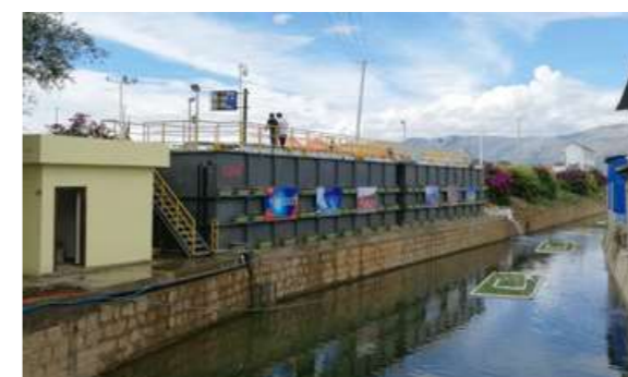
FMBR container for domestic wastewater
