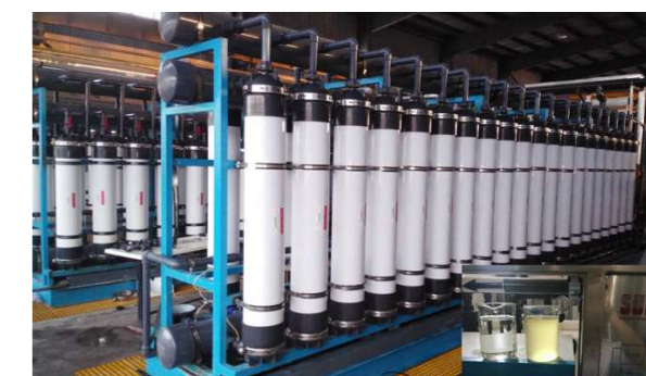
SMBR for industrial wastewater
