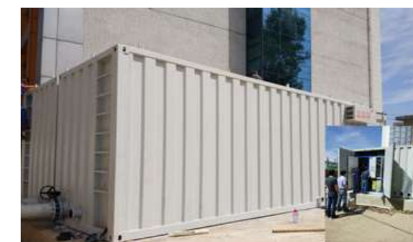
SMBR container for industrial wastewater
